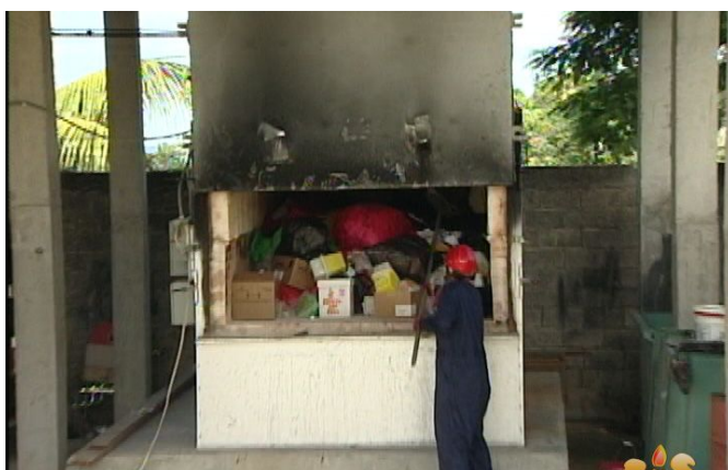
Photo 5.3 Biomedical Waste Gasification Unit
